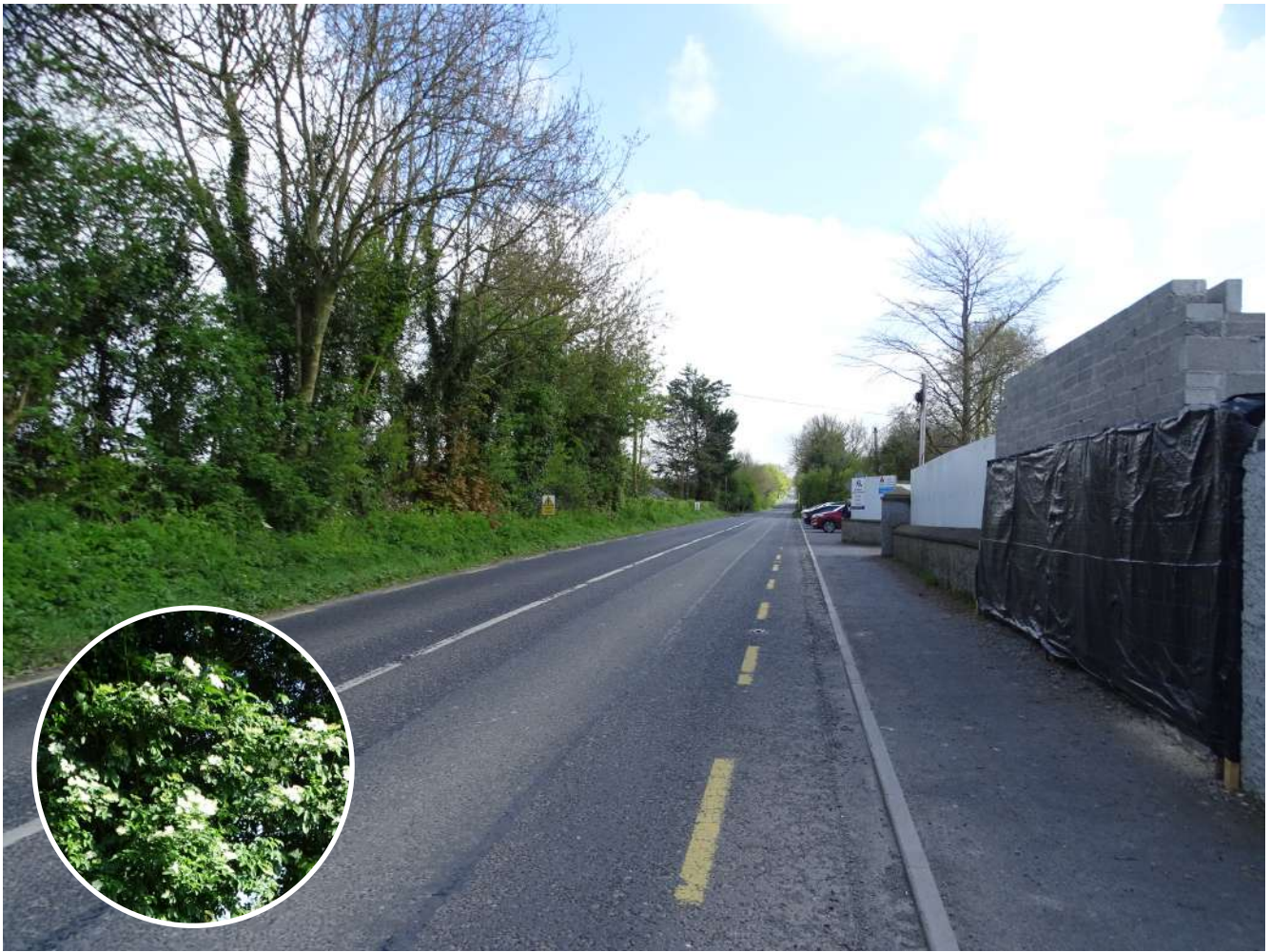
Plate 32: Looking north east along the R418 in Ballyshannon. The private dwelling construction site, the Community Hall and the cars parked outside the school are seen on the right hand side. The road side verge, the hedge and treeline are seen on the left hand side. The hard surface path can be seen on the right hand side. The photo inset shows elderberry in flower in the hedge in June. Photos: © C. O'Connell
