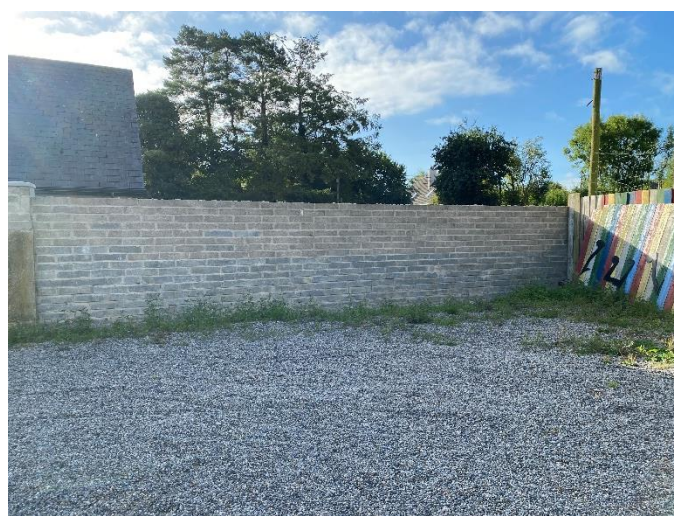
The wall in the back of the community centre could be used to highlight local biodiversity with a mural and combined with native climbing plants
