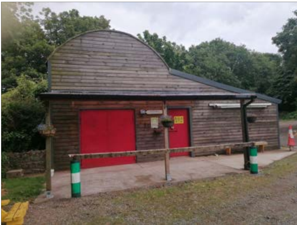
Plate 46. Timber cladding such as that found on the 'Men's Shed' can provide ideal roosting spaces for bats.
