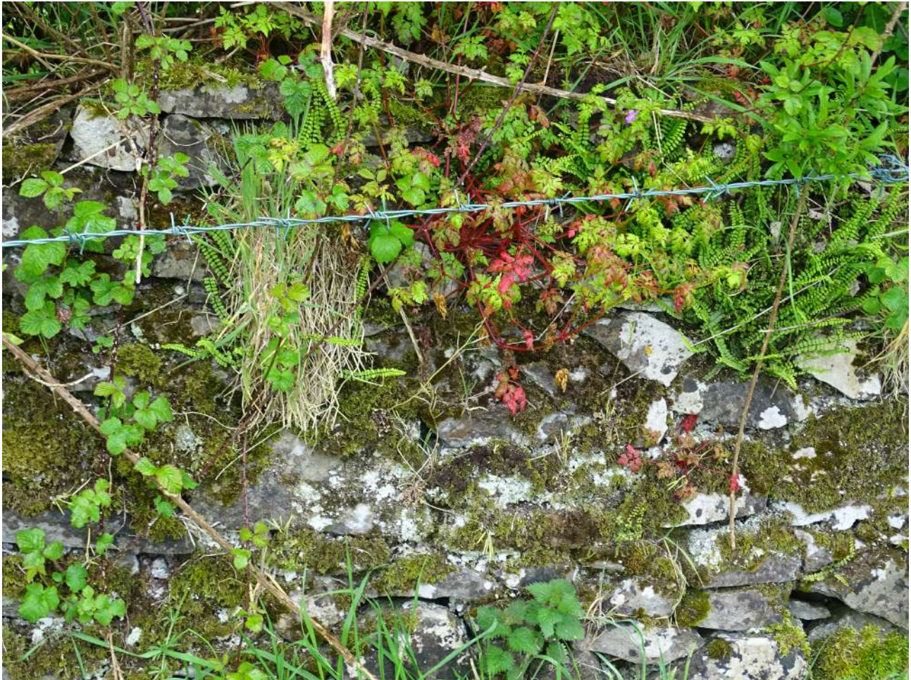
Plate 31: Close up of the stone wall along the lane access to Tobar Mhuire showing the abundance of plants that have colonised it. The nooks and crannies within the wall provide habitat for breeding birds and insects. Action 6.6.2 in Table 9 recommends retaining the walls as they are for biodiversity. Photo: © C. O'Connell
