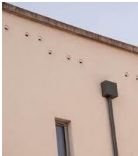
Plate 29: Built-in Swift boxes at Westport Town Hall. Source: Swift Conservation Ireland
