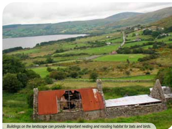
Buildings on the landscape can provide important nesting and roosting habitat for bats and birds.
