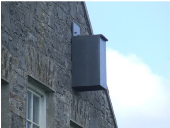
Figure 14: Bat box on the east wall of St. Patrick's Hall, Ballacolla, Co. Laois
