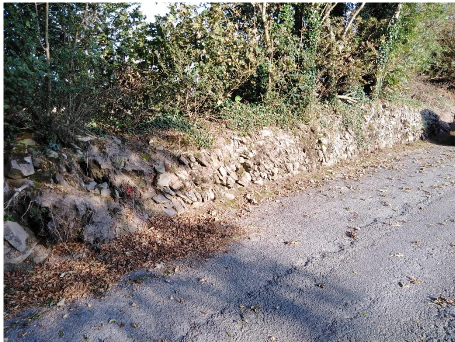
Fig. 11 Sprayed section of stone breasted bank and subsequent collapse of part of it
