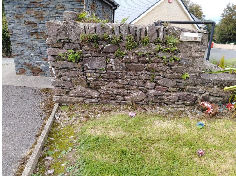
Fig. 15 Section of wall colonised by hart's tongue fern, wall rue and black spleenwort species of fern
