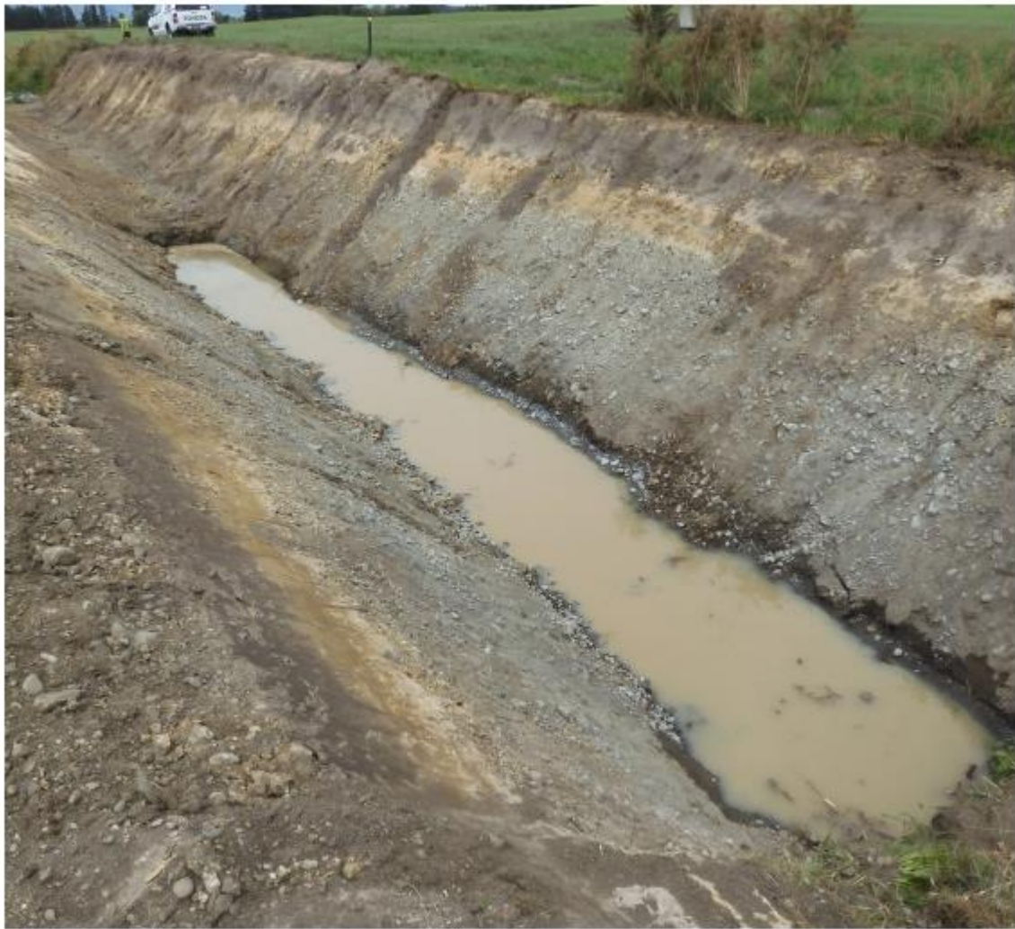
Figure 34. In stream works with a sump to trap sediment by gradual reduction in water velocity for its length
