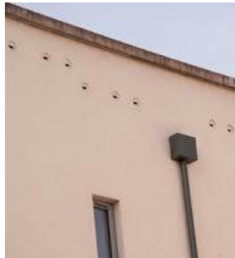
Plate 2: Built-in Swift boxes at Westport Town Hall. Source: Swift Conservation Ireland
