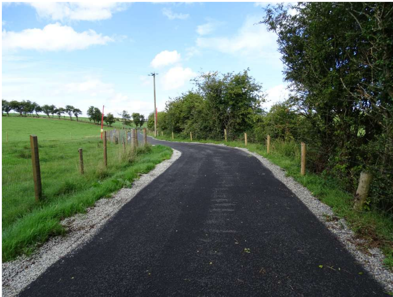
Plate A: view of the new cycle route adjacent to Belleek woods. The agricultural land to the left has been fenced off as has the hedgerow to the right hand side in the photograph. The sides of the route are dressed with loose stones onto which grasses are colonising. Photo: © C. O'Connell.
