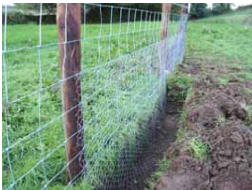
This sturdy fence will protect trees from livestock. Note the rabbit wire buried and bent outwards
